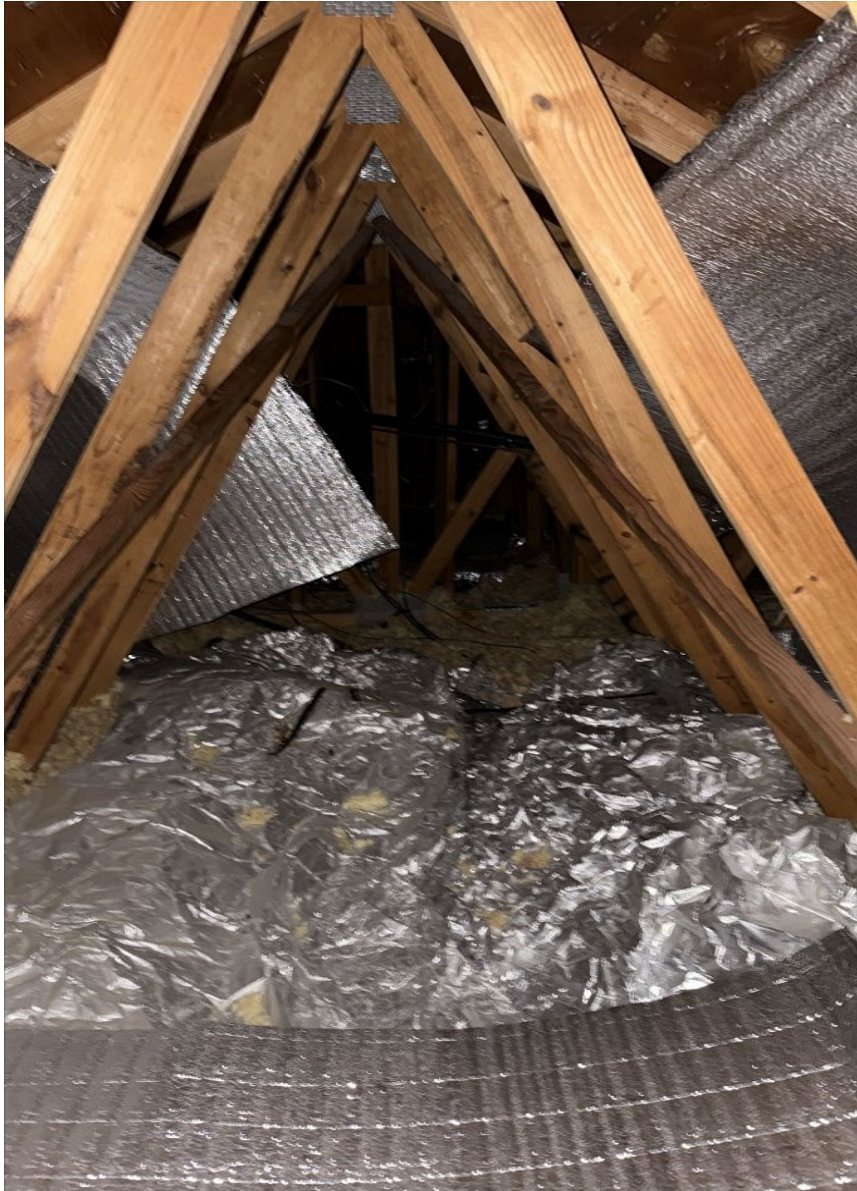
Figure 11-5: Ceiling Insulation Project- No Insulation Installed Due to Radiant Barrier
