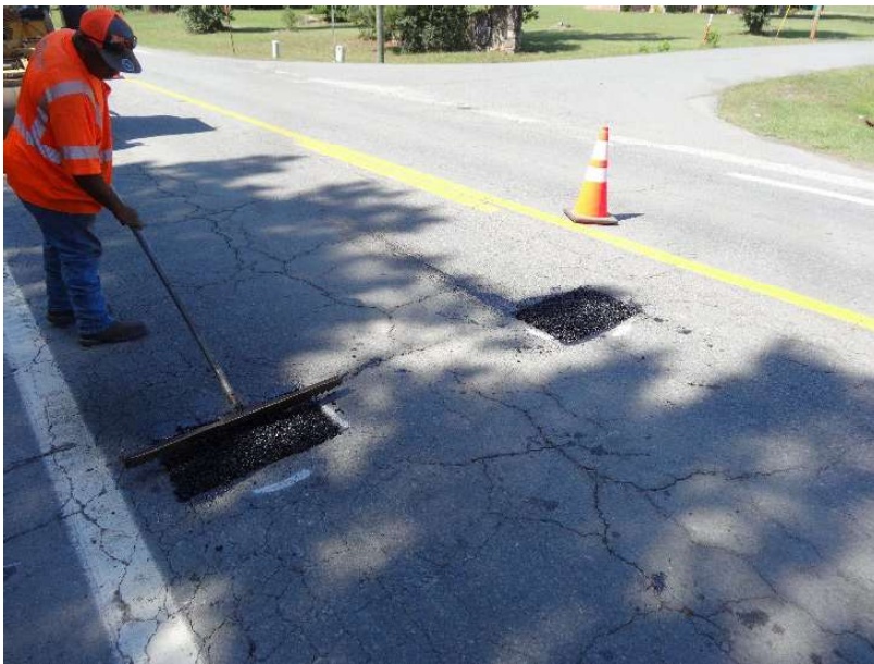
Figure 10. Overfilled Repair Materials Before Compaction
