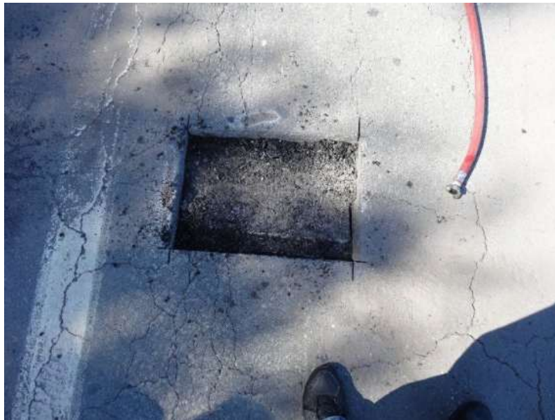
Figure 6. Rectangular Pothole After Cleaning
