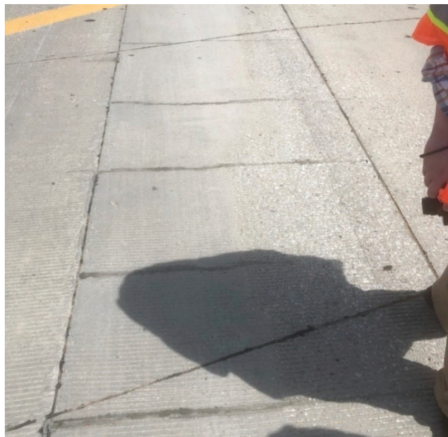
Figure 1. Transverse Cracking on Concrete Bridge Deck Surface
