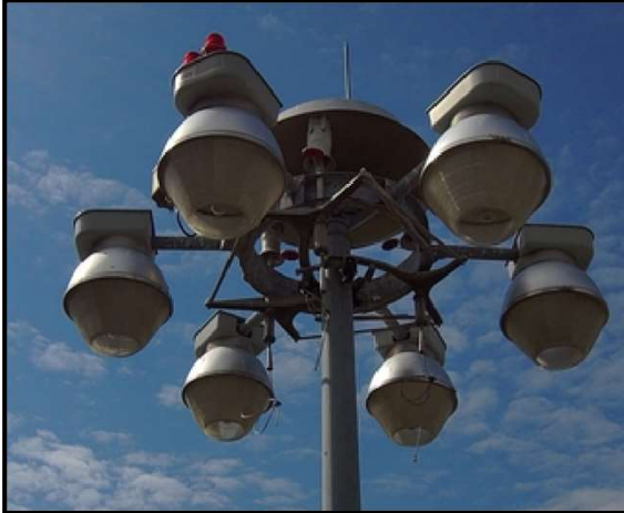
High Pressure Sodium
