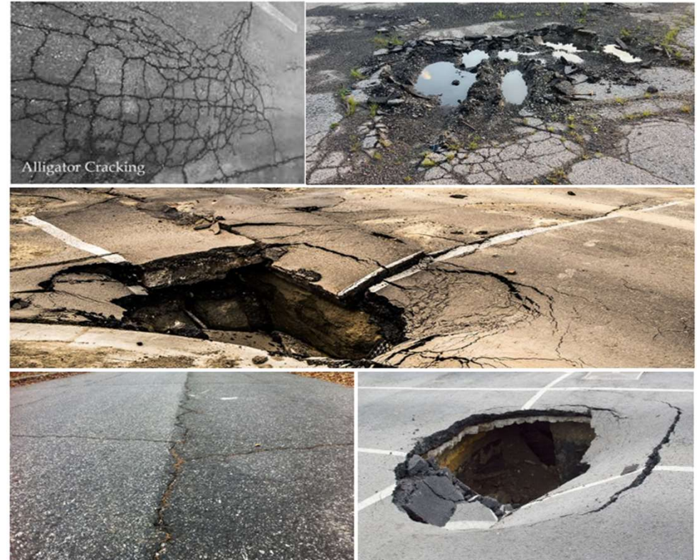
Example Pavement Failures Due to Weak Subgrade Soils
