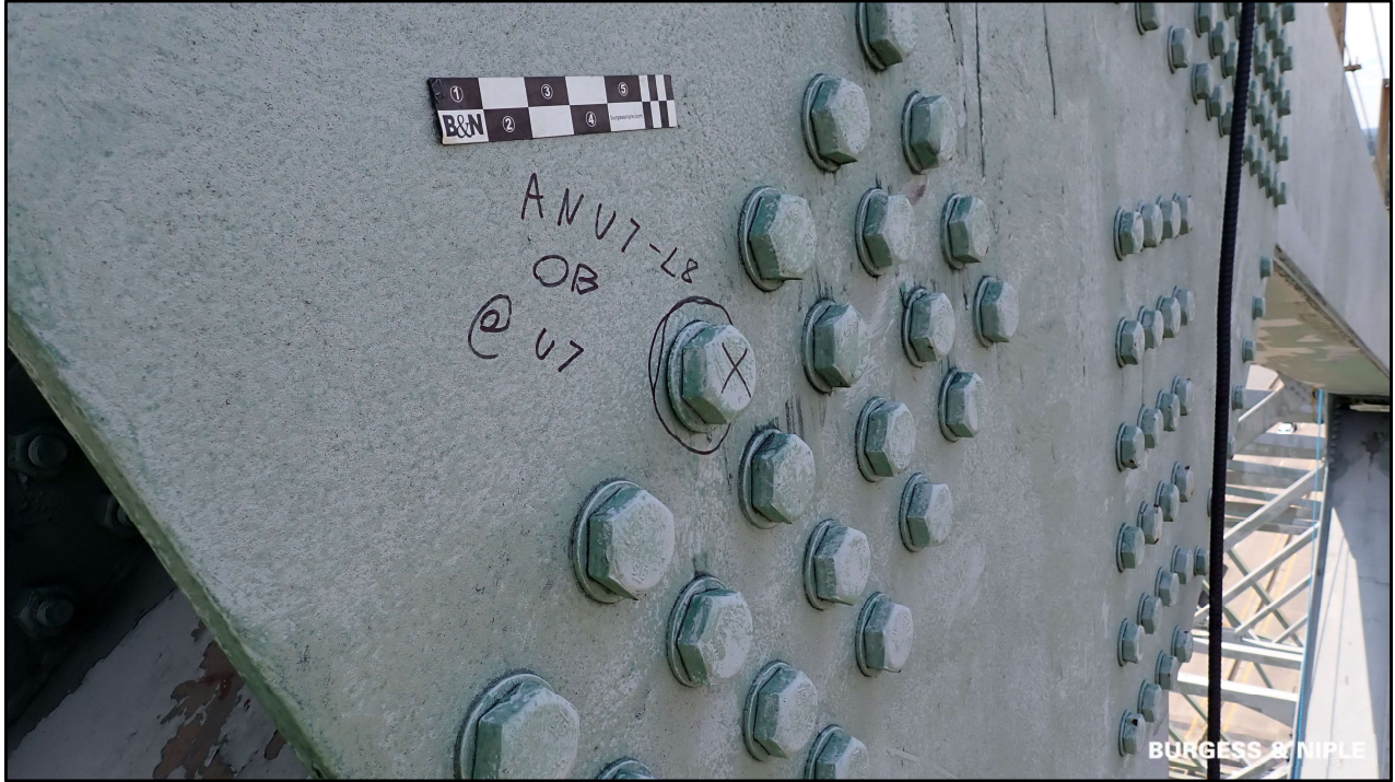
With out the maker on the bolt there is no way a drone would be able to tell that washer is loose.
