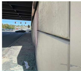
Bowing of the wall
