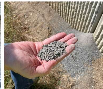
Loss of backfill
