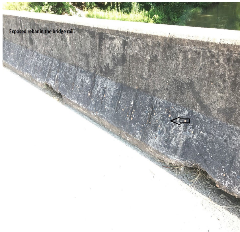
Figure 14. Exposed rebar in the bridge rail.
