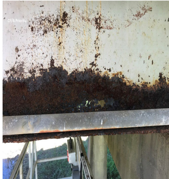
Figure 26. CF/A priority on steel girder end
