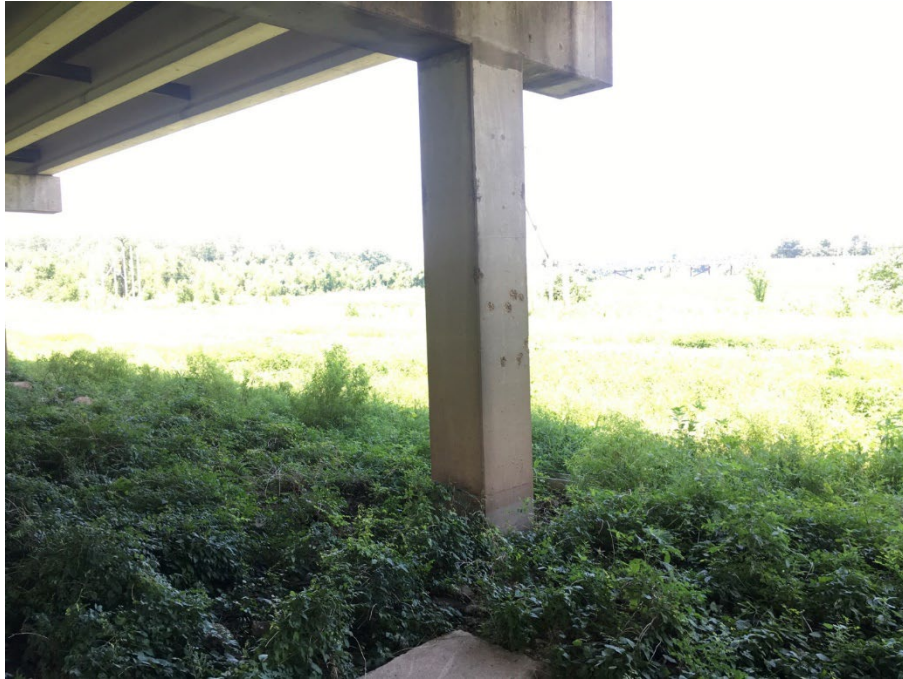
Figure 6. Good example of small spalls from gun shots that does not need to be a maintenance need
