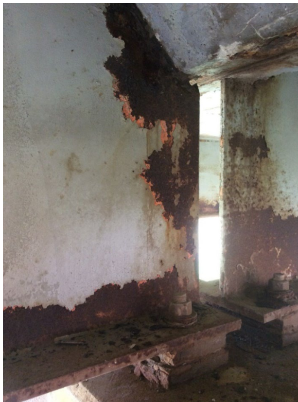
Figure 32. C/D priority of Steel Girder End
