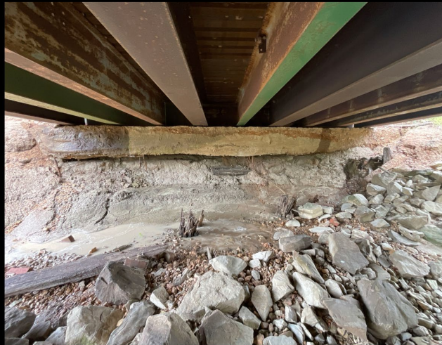
Bent 2 scour up to 2'-7" down and 3' back under 5-12-2025
