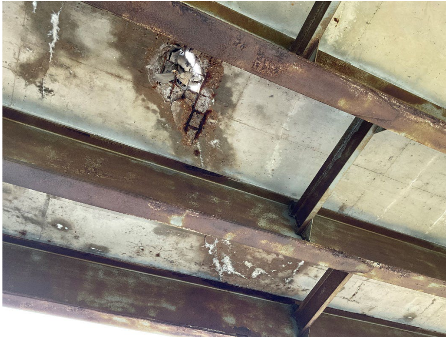
Figure 36. CF or A on the deck – full depth hole that needs full depth patch
