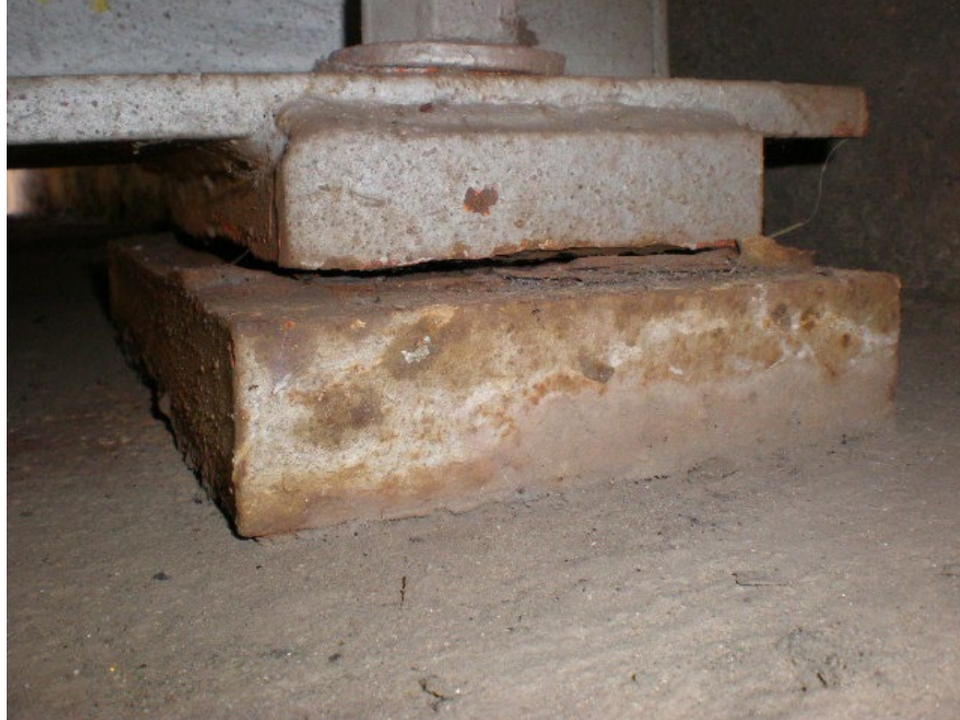
Figure 1. Good example for: A-57 - Beam End and Bearing Painting Needed – No need for maintenance need
