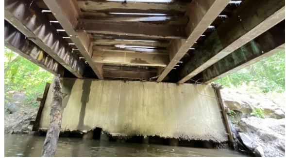
Figure 1 Undermining of the abutment exposing piles.
