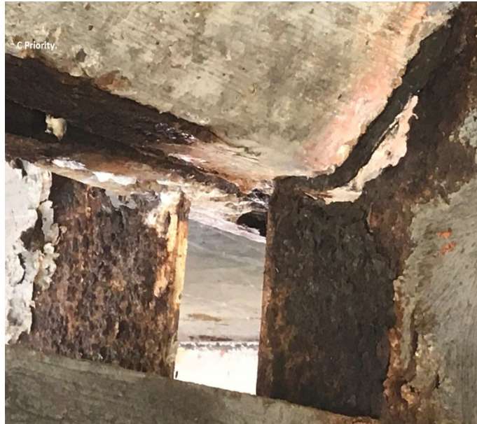
Figure 27. C priority on steel girder end
