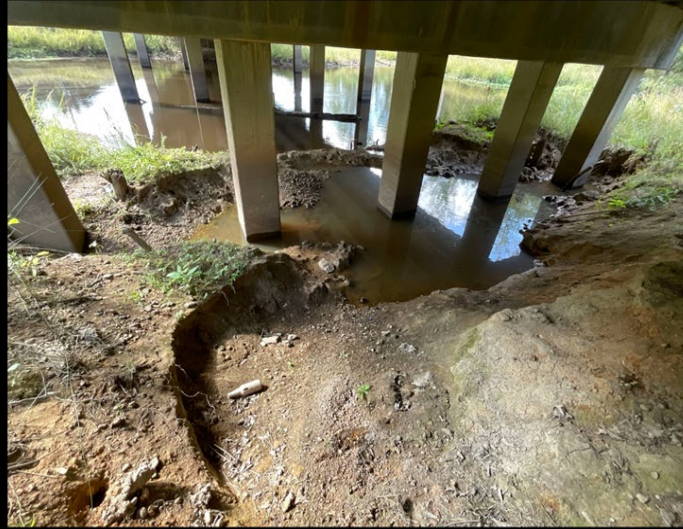
Isolated moderate scour around bent 5.
