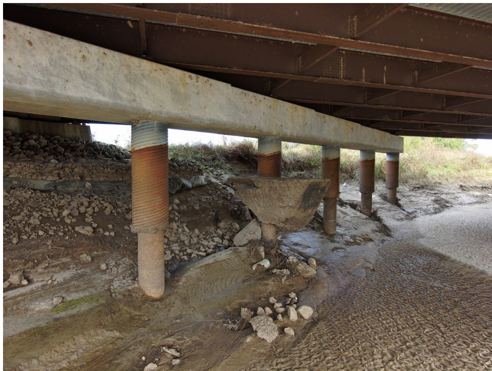
Figure 43. B Priority (depending on depth of piles or shafts). Needs to be evaluated by an engineer for depth of pile fixity
