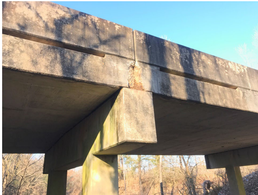
Figure 18. Spall on exterior face of concrete slab
