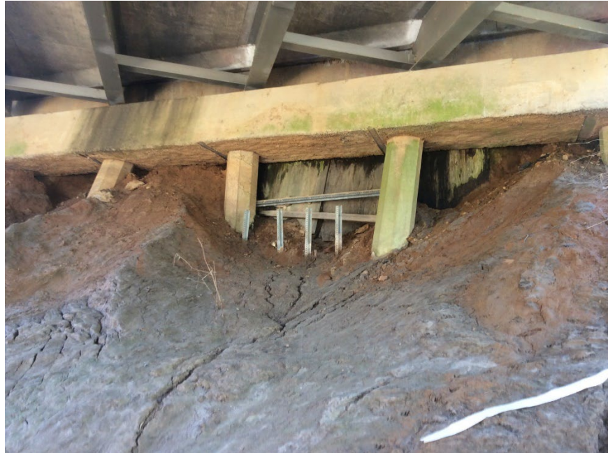
Figure 42. A Priority of multiple piles exposed at the abutment with material behind abutment spilling through. Needs Engineering review.
