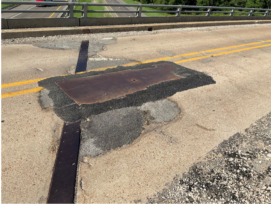
Figure 37. B priority since the plate is in place. Full depth deck patch needed
