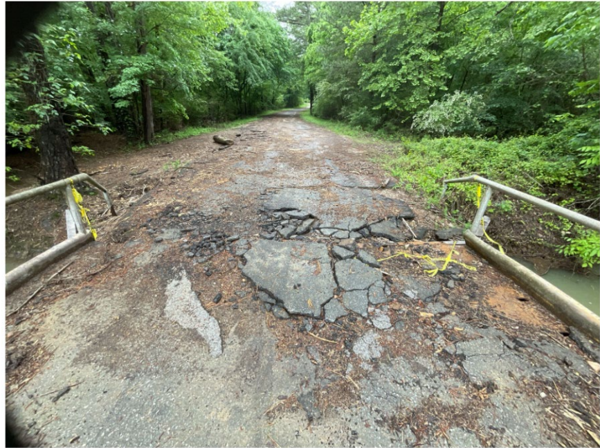
West approach has been washed out
