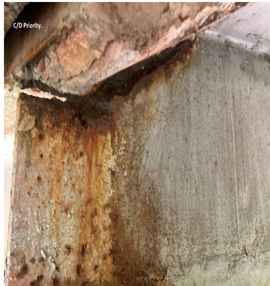
Figure 25. C/D priority of steel girder end
