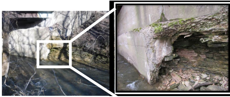
Figure 5 Bridge with non-scour-resistant rock.
