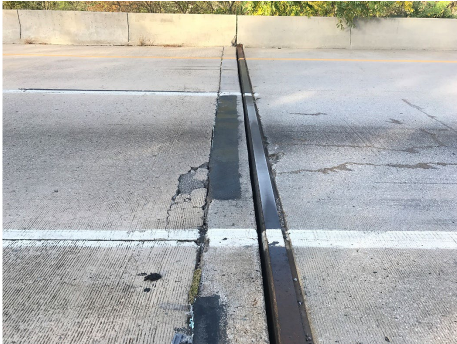
Figure 45. B/C priority of delamination/spalled area that needs to be addressed in a timely manner. Also pictured: a joint seal that can be taken care of with a check box maintenance item.
