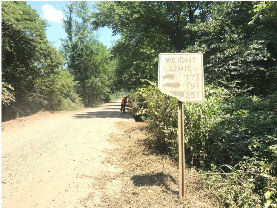
Figure 49. B priority maintenance need for other posting issue where sign is damaged and covered in debris making it hard to read.
