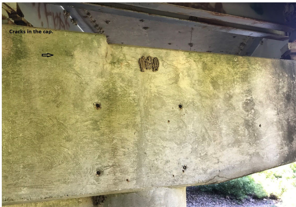
Figure 22. Minor cracks in top of caps
