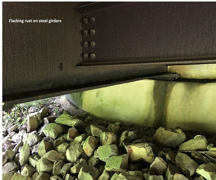
Figure 20. Flaking rust on steel girders. Can be covered with check box maintenance item.
