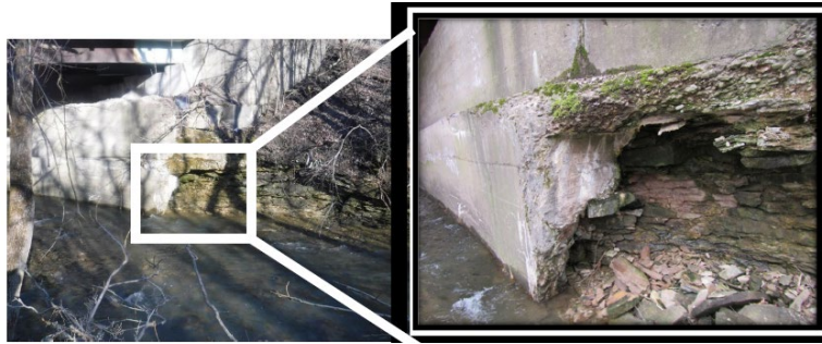
Figure 5 Bridge with non-scour-resistant rock.
