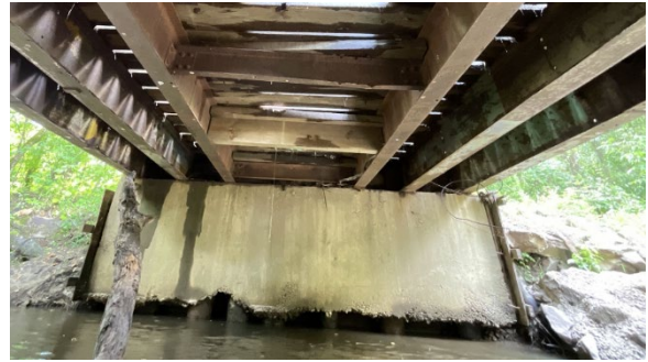
Figure 1 Undermining of the abutment exposing piles.
