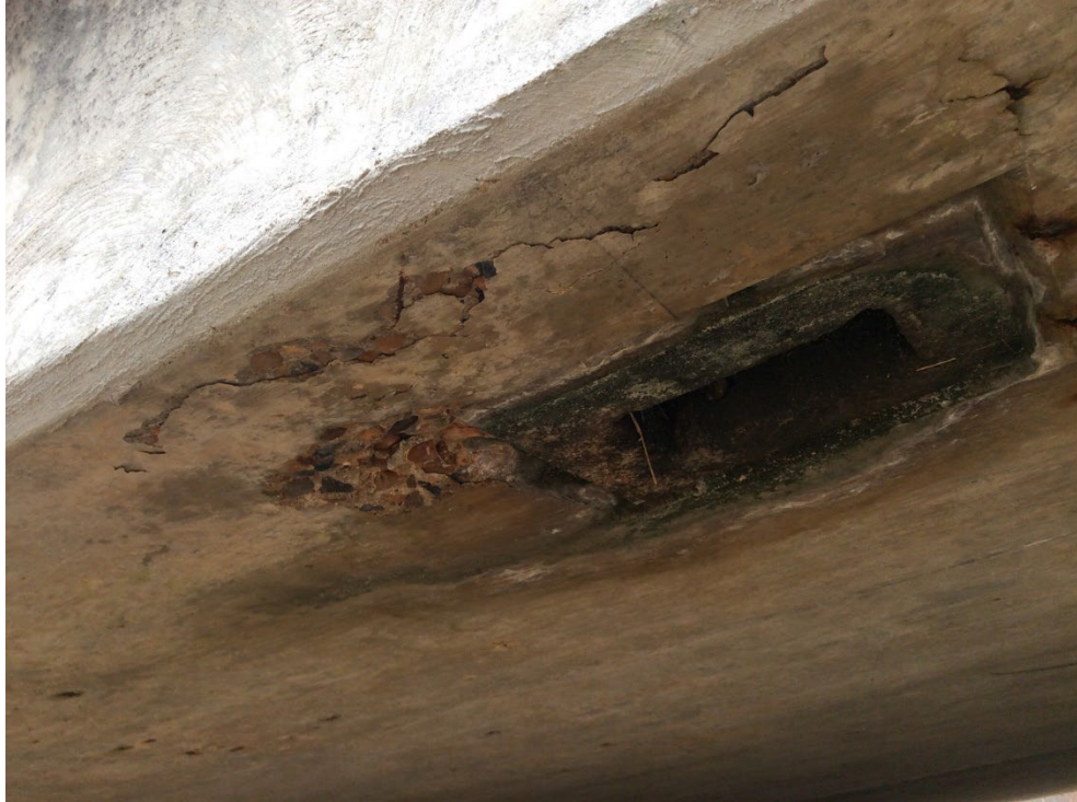
Figure 19. Delaminated concrete around drains
