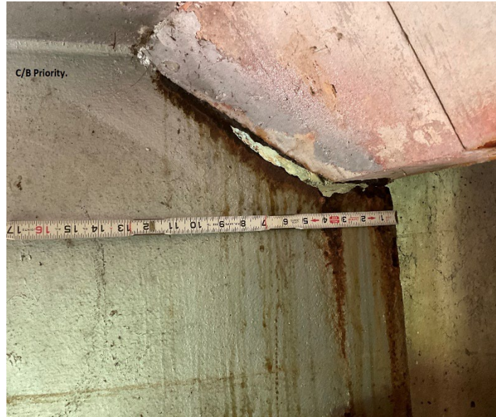
Figure 31. C/B priority on Steel Girder End section loss at haunch area
