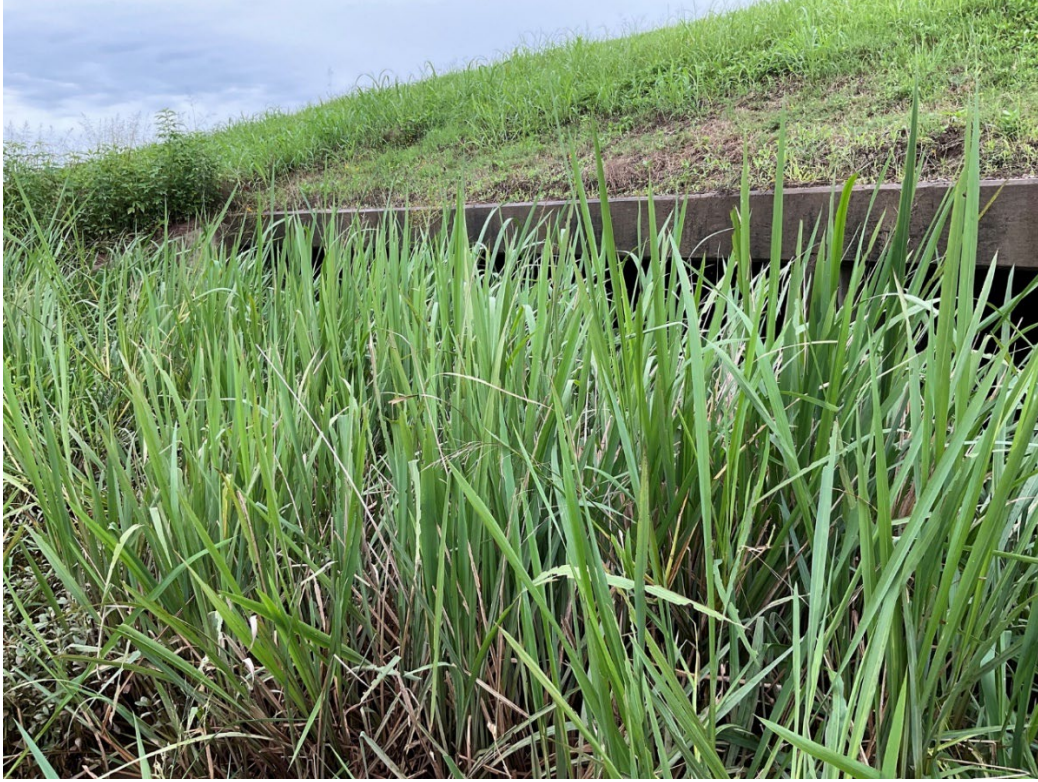
Figure 5. C/D priority maintenance item for vegetation.
