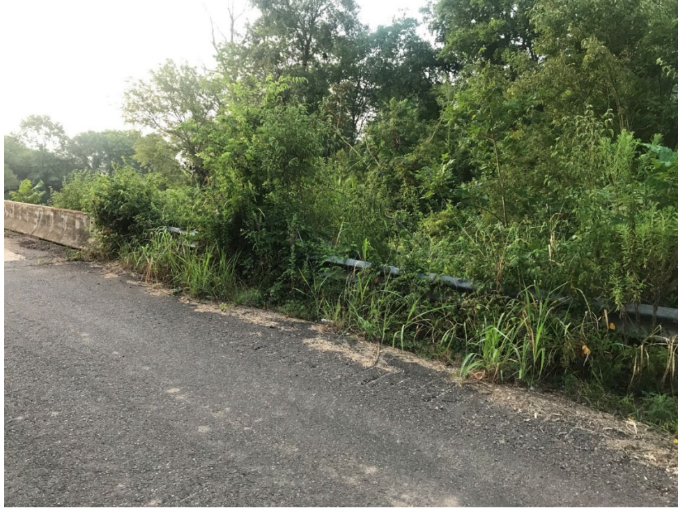
Figure 3. C/D priority maintenance item for vegetation.
