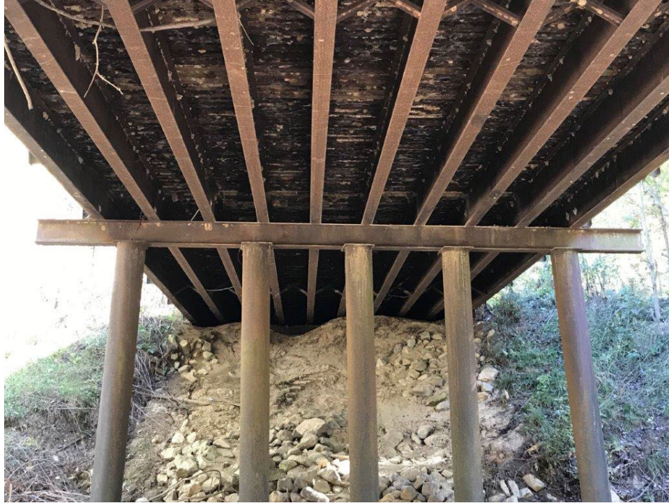
Figure 7. Good example of check box maintenance need for full beam painting
