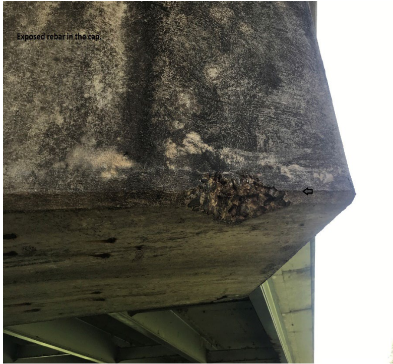
Figure 17. Minor Spall on cap
