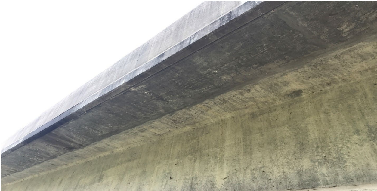
Figure 8. Example of efflorescence cracking in the overhang that does not need to be a maintenance need. Document in the element quantities.
