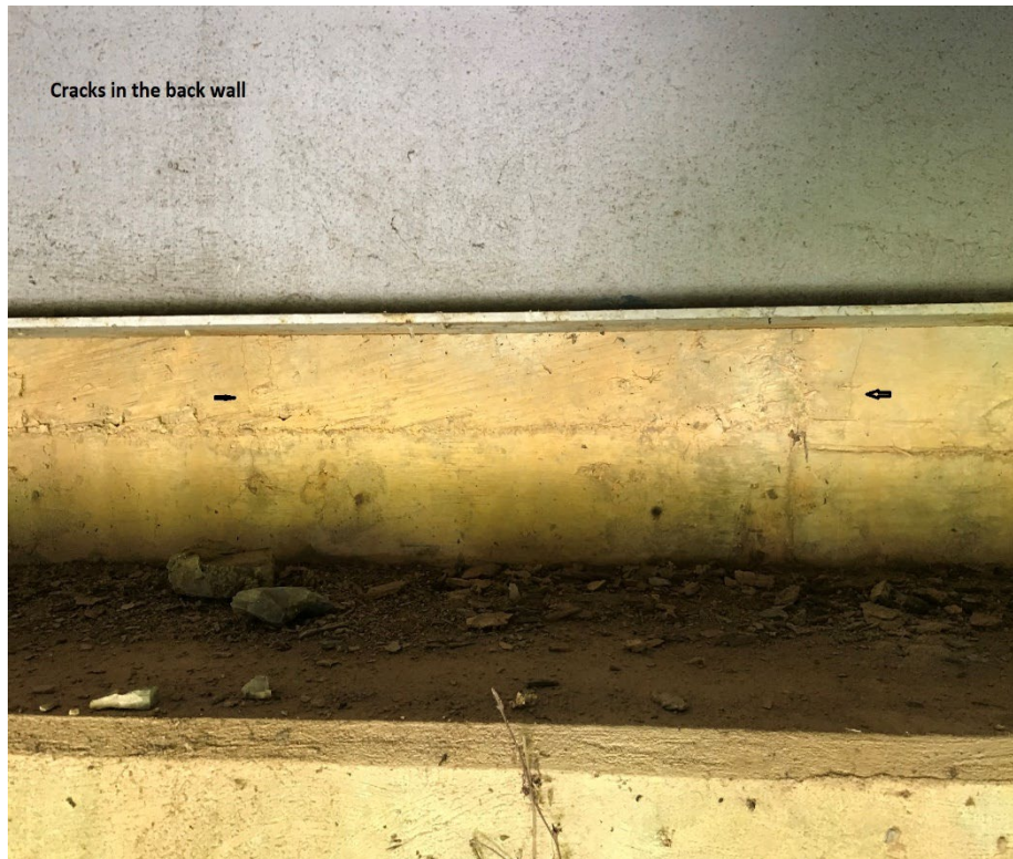
Figure 15. Minor cracks in the back wall
