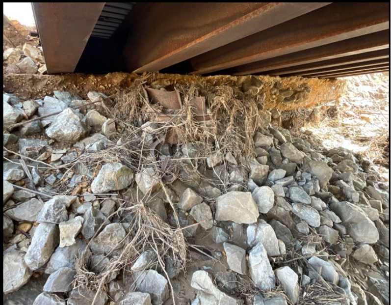
Bent 1 is up to 2.5' undermined from centerline to left end 4-28-2025
