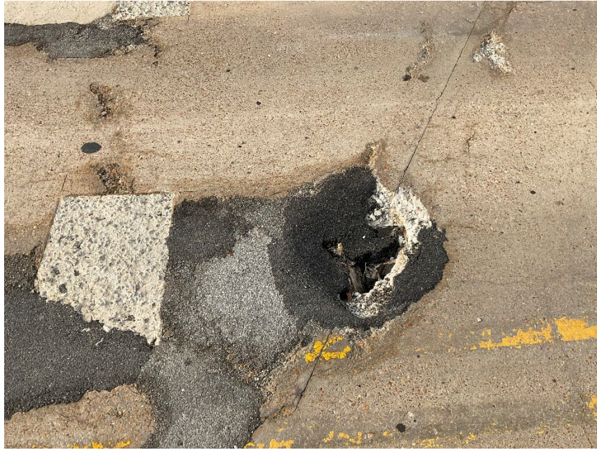
Figure 35. CF priority on the deck – full depth hole that could cause wreck
