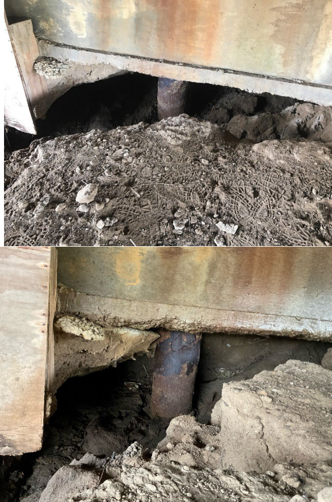
Figure 41. Photos of A/B priority of erosion under pile cap with steel shell pile exposed and adjacent concrete exposed.
