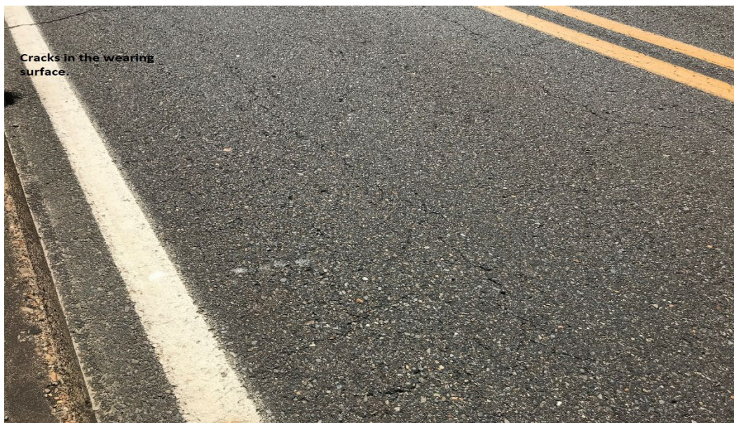
Figure 10. Cracks in wearing surface that should not be a maintenance need.
