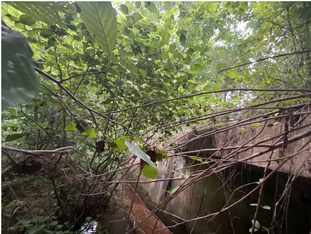
Figure 4. C priority maintenance item for vegetation. If access is 100% limited code a B priority.
