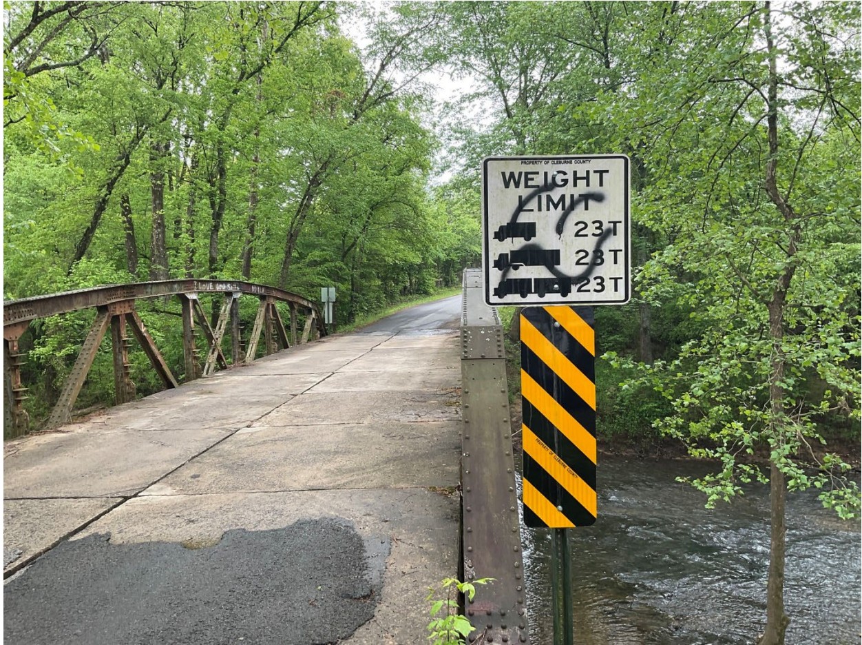
Figure 52. B priority maintenance item for sign vandalism.
