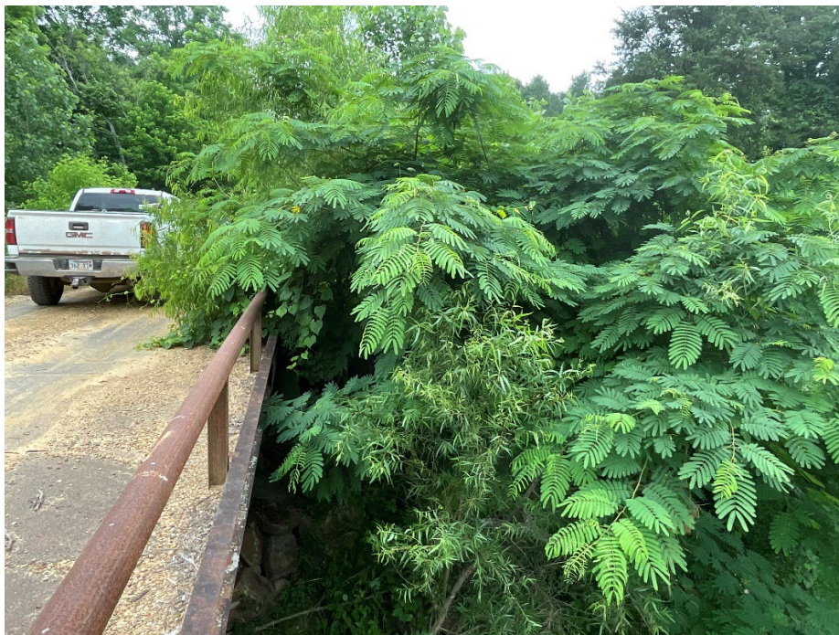
Figure 2. C/D priority maintenance item for vegetation.
