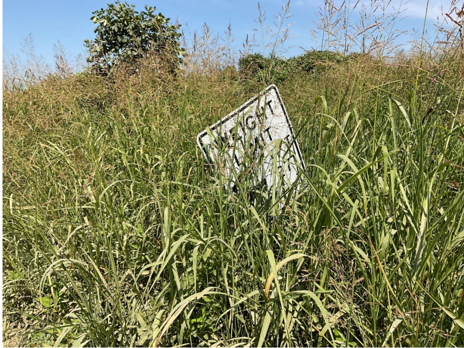
Figure 48. B priority maintenance need for other posting issue where vegetation is partially obstructing signage
