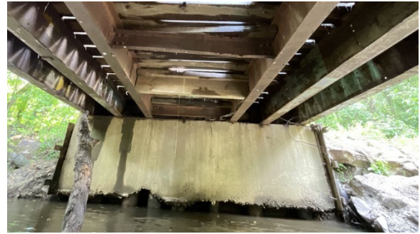
Figure 1 Undermining of the abutment exposing piles.
