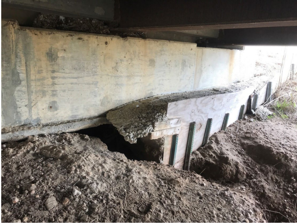
Figure 44. B/C priority of area that continues to erode from under the concrete cap.
