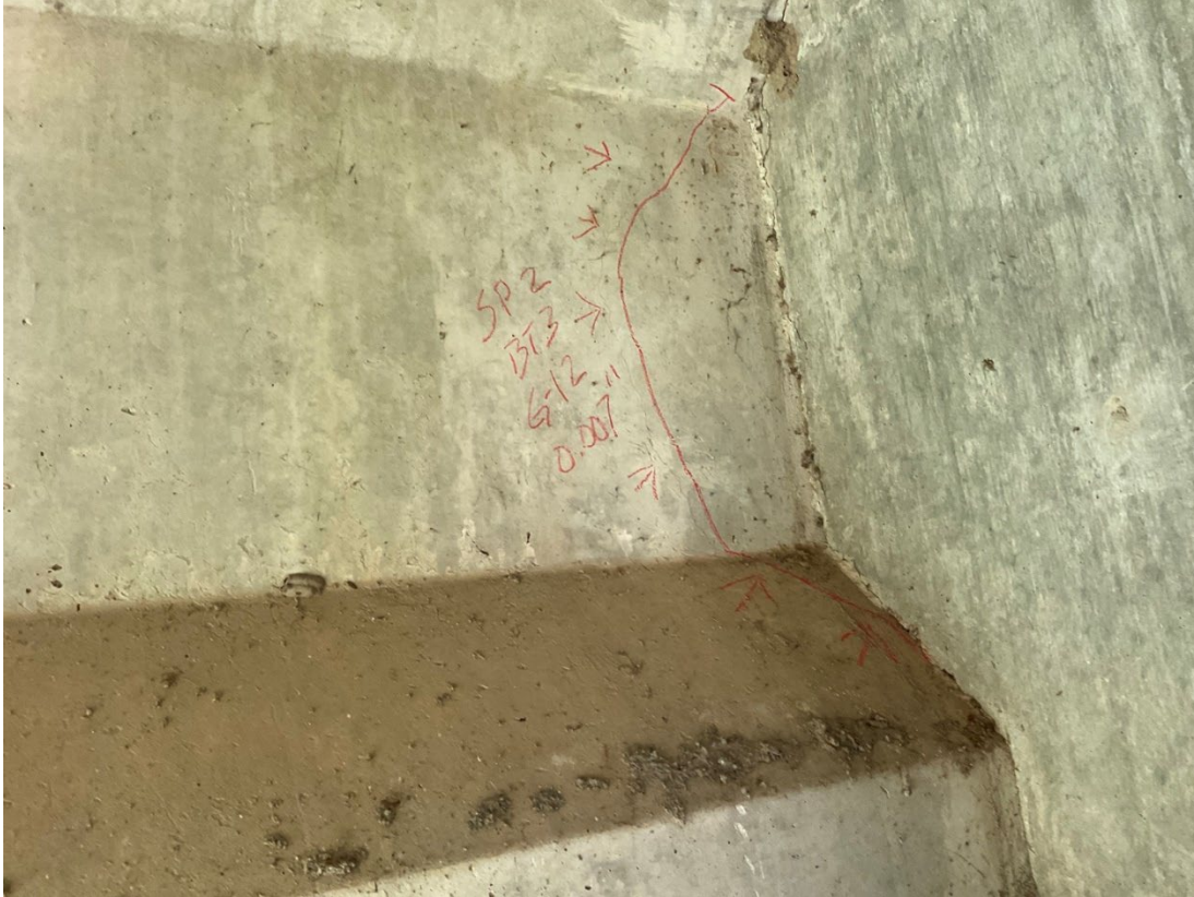
Figure 9. Prestressed girders with diagonal or vertical crack (non-shear cracks) less than CS2 that do not need to be a maintenance need. CS3 or worse would need to be maintenance
