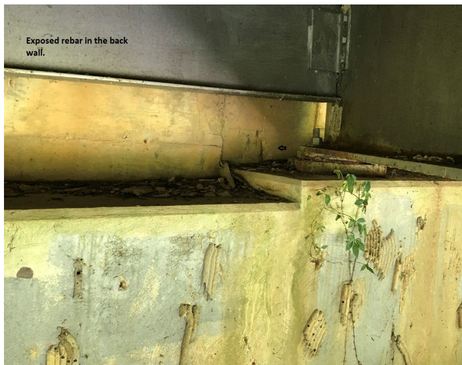
Figure 16. Small area of a single exposed bar in the back wall
