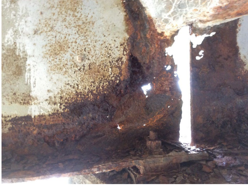
Figure 34. CF priority of Steel Girder end with crushing action
