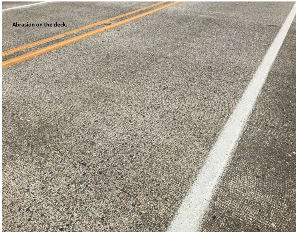
Figure 21. Abrasion on concrete deck
