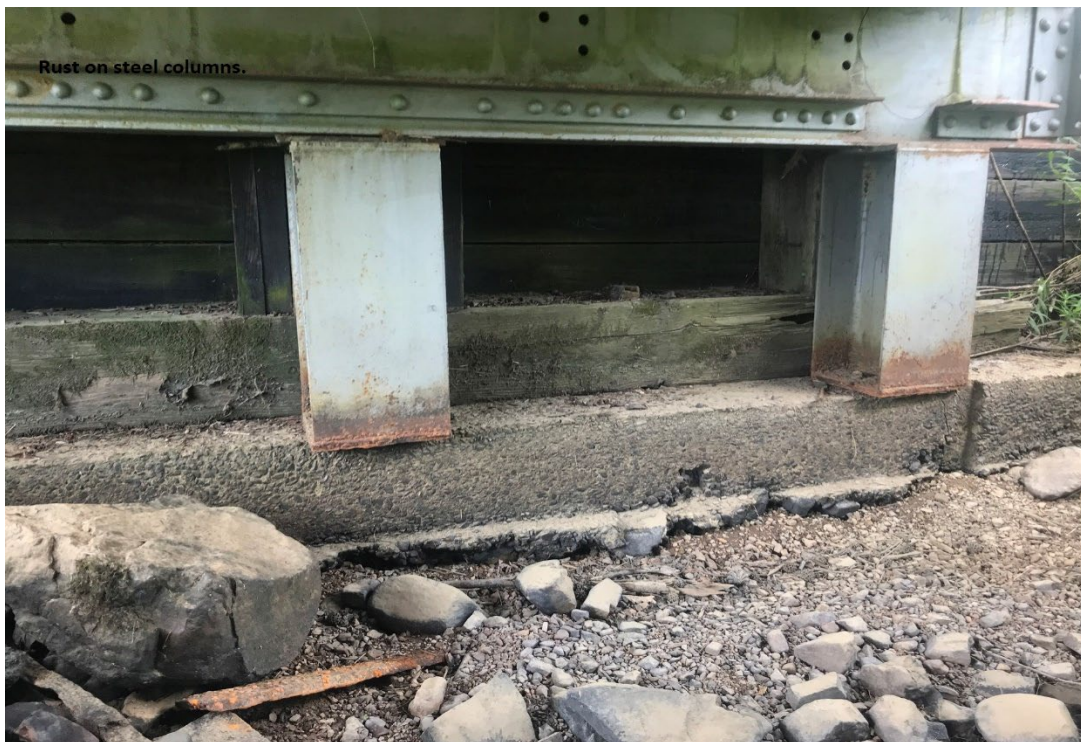
Figure 24. minor localized rust of steel columns. Note: rust and section loss on steel at concrete connections (like piles into caps) should be a maintenance need.
