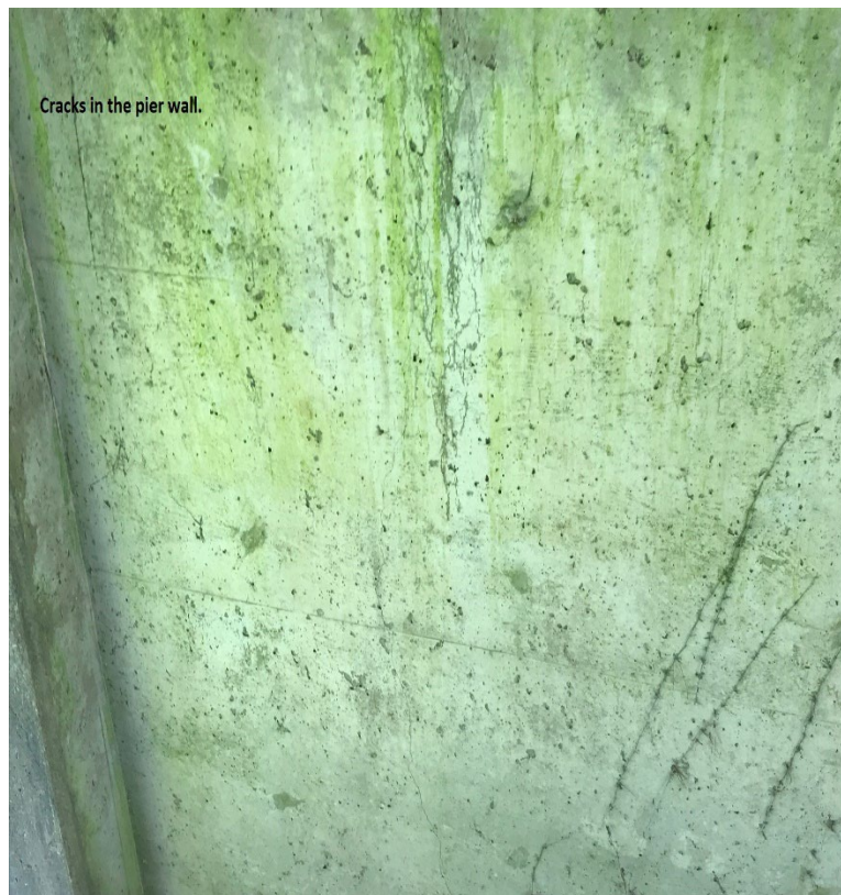
Figure 12. Minor cracks in the pier wall
