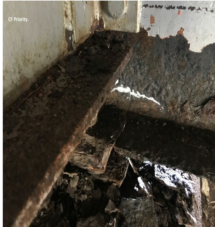
Figure 29. CF priority on Steel Girder end with crack through bottom flange
