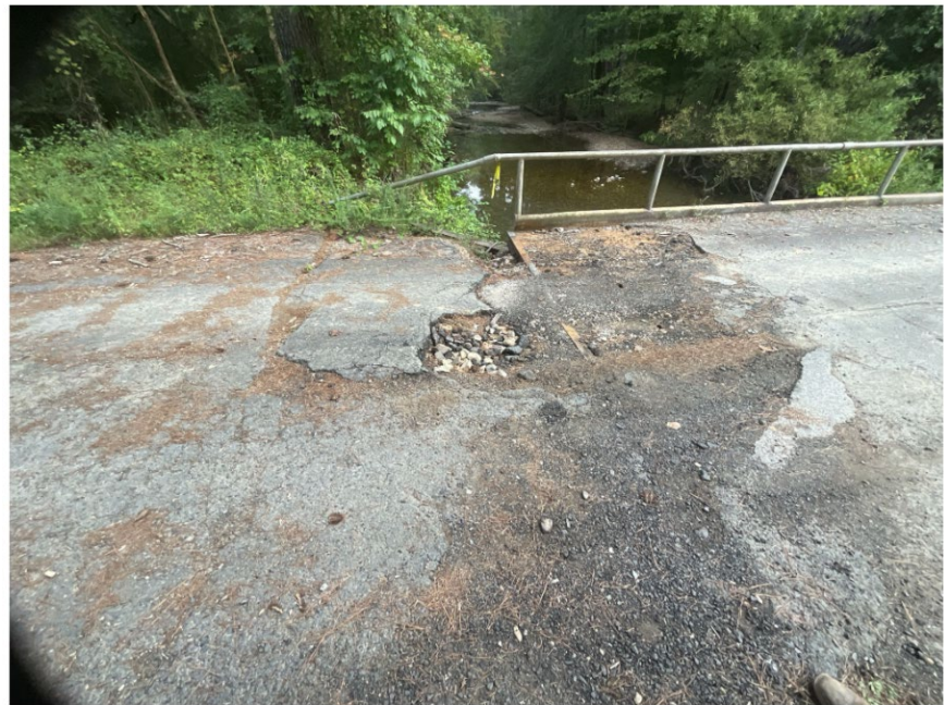
Approach roadway washed out no repairs have been made
