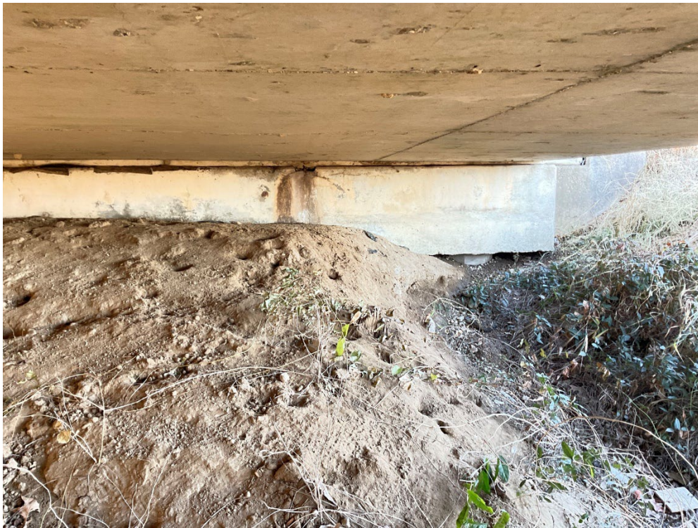
Figure 40. C priority of erosion under pile cap/abutment
