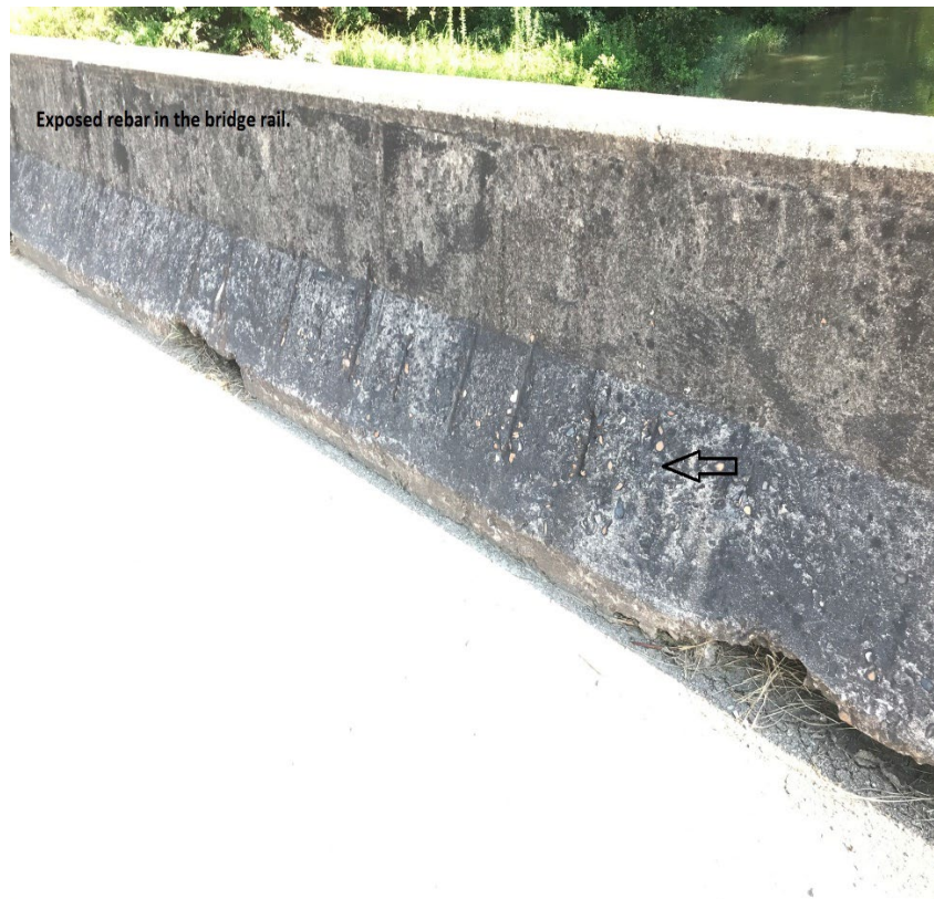
Figure 14. Exposed rebar in the bridge rail.
