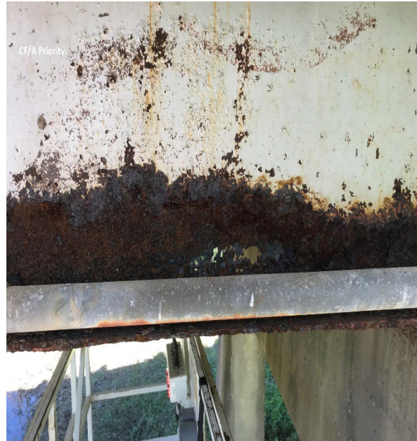
Figure 26. CF/A priority on steel girder end
