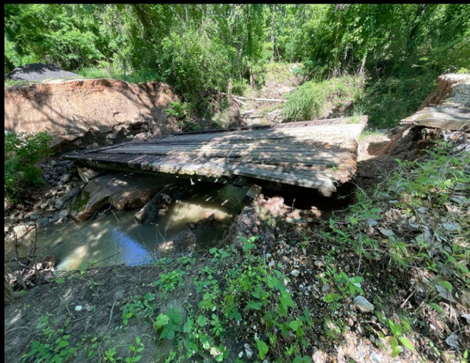
Bridge has failed and is closed.
