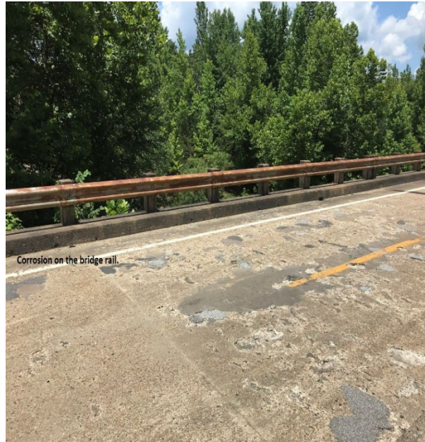
Figure 13. Corrosion on the bridge rail. Note: the deck shown should have a maintenance need
