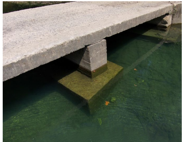
Figure 2 Exposed footing with undermining.
