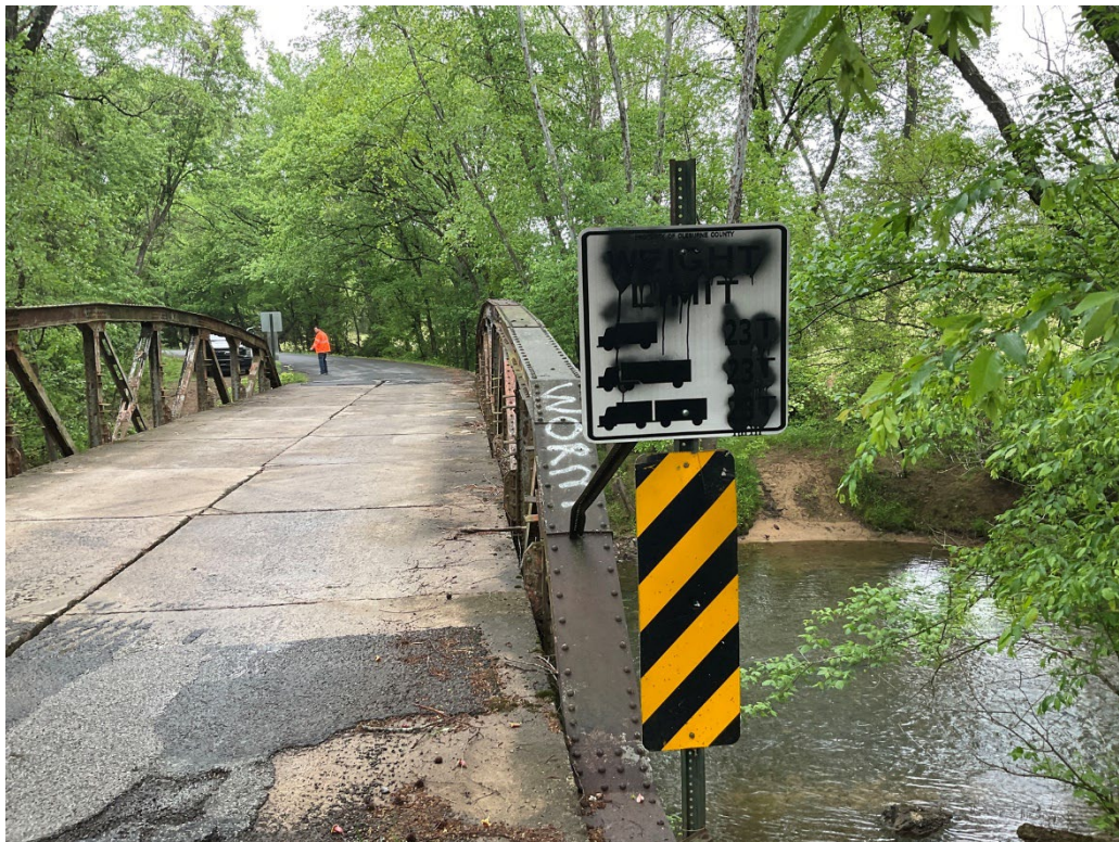
Figure 51. A priority maintenance item for posting sign vandalism.
