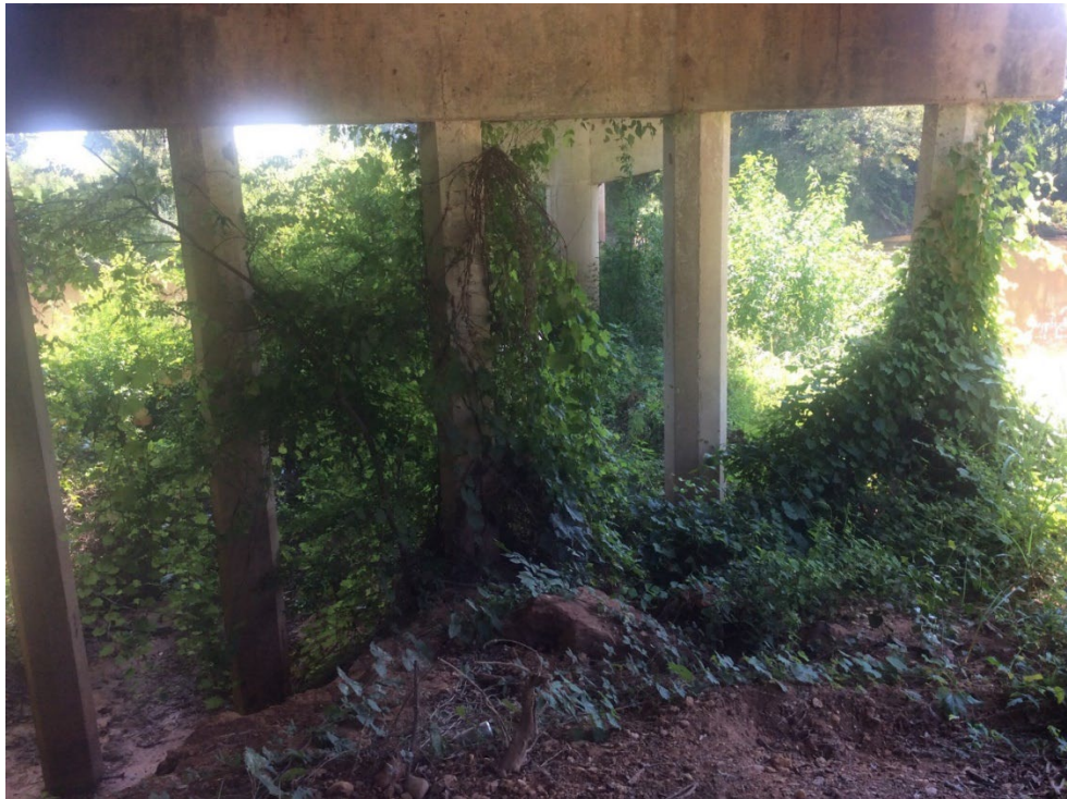
Figure 8. D priority maintenance item for vegetation due to limiting inspection.
