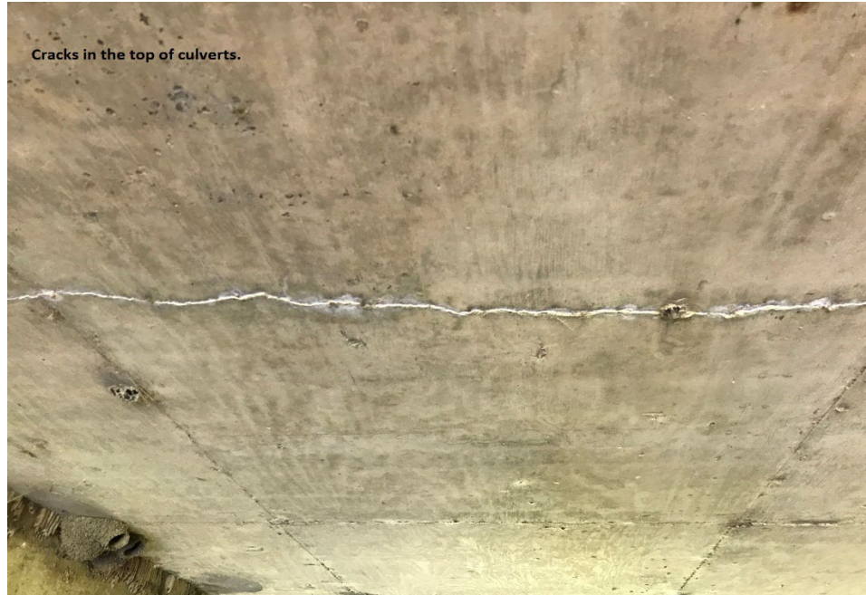
Figure 23. Cracks in top of culverts. Document defect in defect quantities and note in the corresponding element or component (based on owner).
