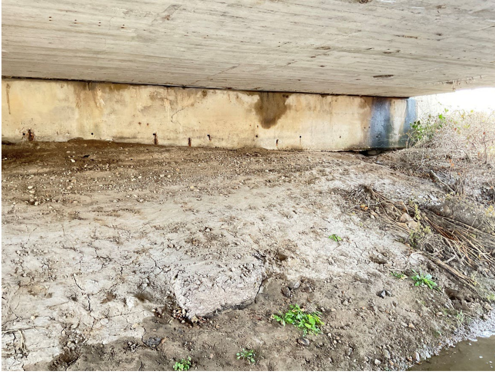
Figure 39. D priority of erosion under pile cap/abutment
