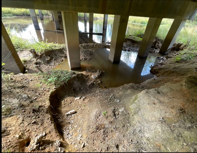
Isolated moderate scour around bent 5.
