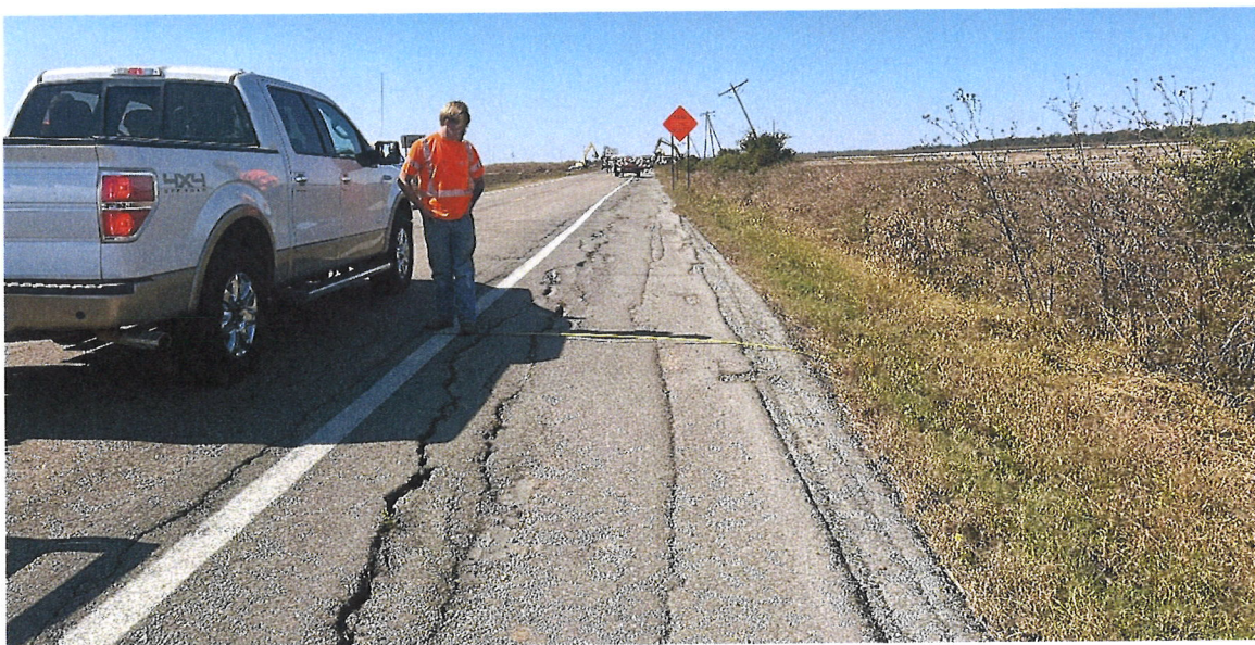
Shoulder failure north side of road looking west.
