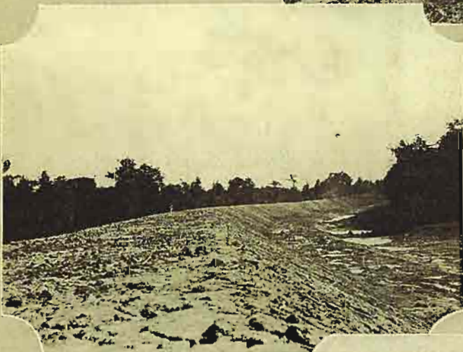
Excellent example of dragline work on new location of Route No. 167, northeast of Camden.
