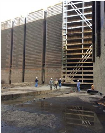
Dewatering the Dardanelle Lock & Dam (L&D No. 10), MKARNS in Russellville, AR (2017). Image Source: ARDOT.
