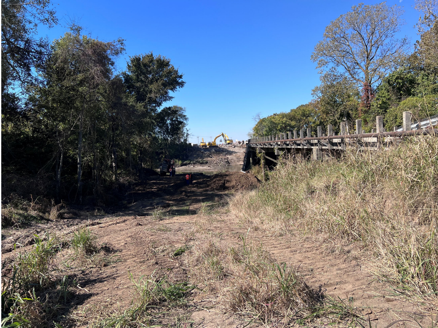
South side of east bridge end looking west (Late October 2024 During Demolition)
