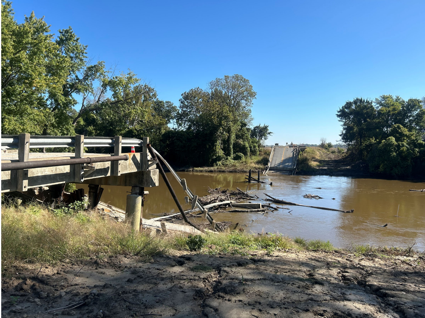
South side of east bridge end looking northeast (Early October 2024 Before Demolition)
