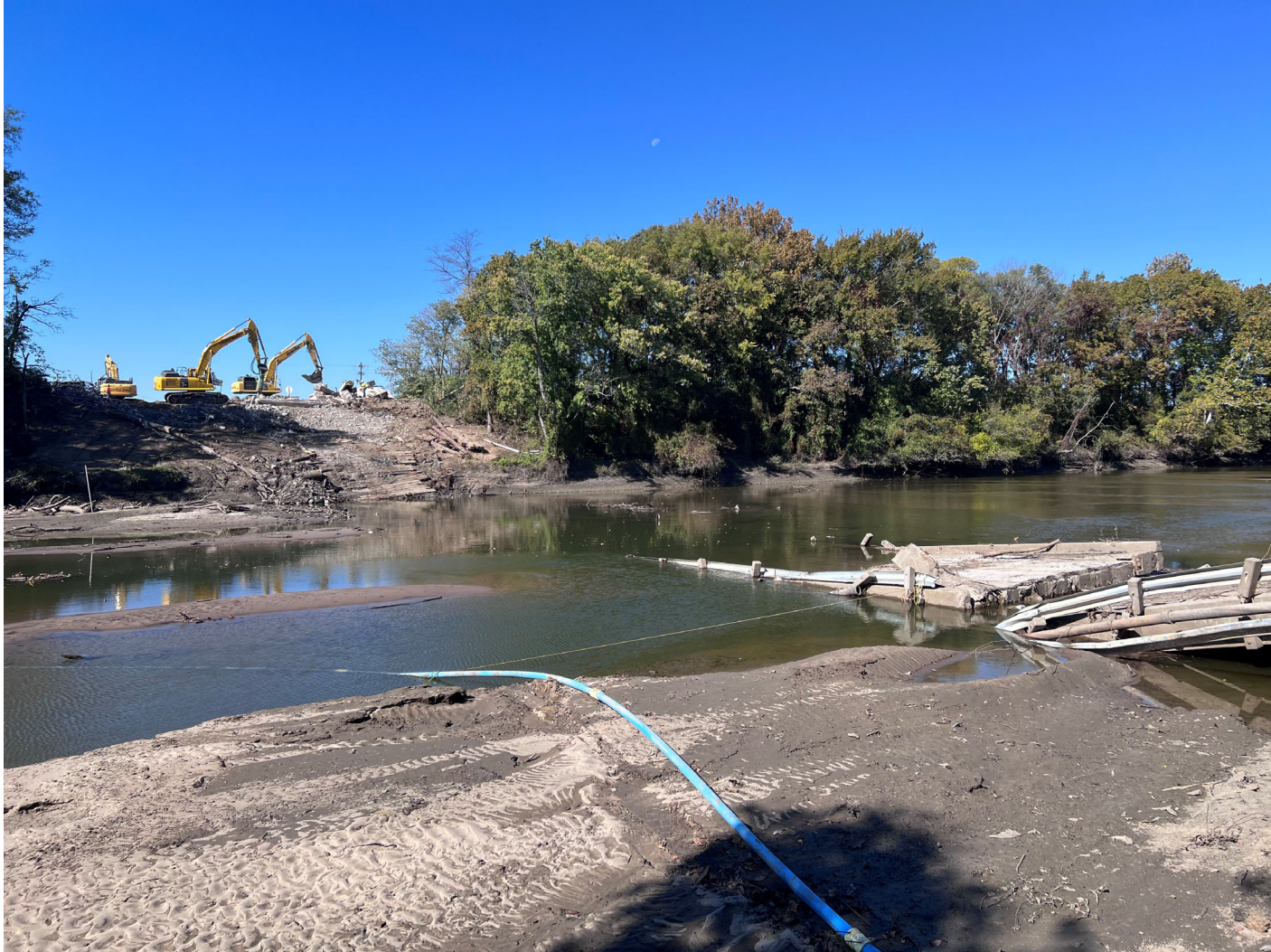
South side of collapsed bridge looking northwest towards west bridge end (Late October 2024 During Demolition)
