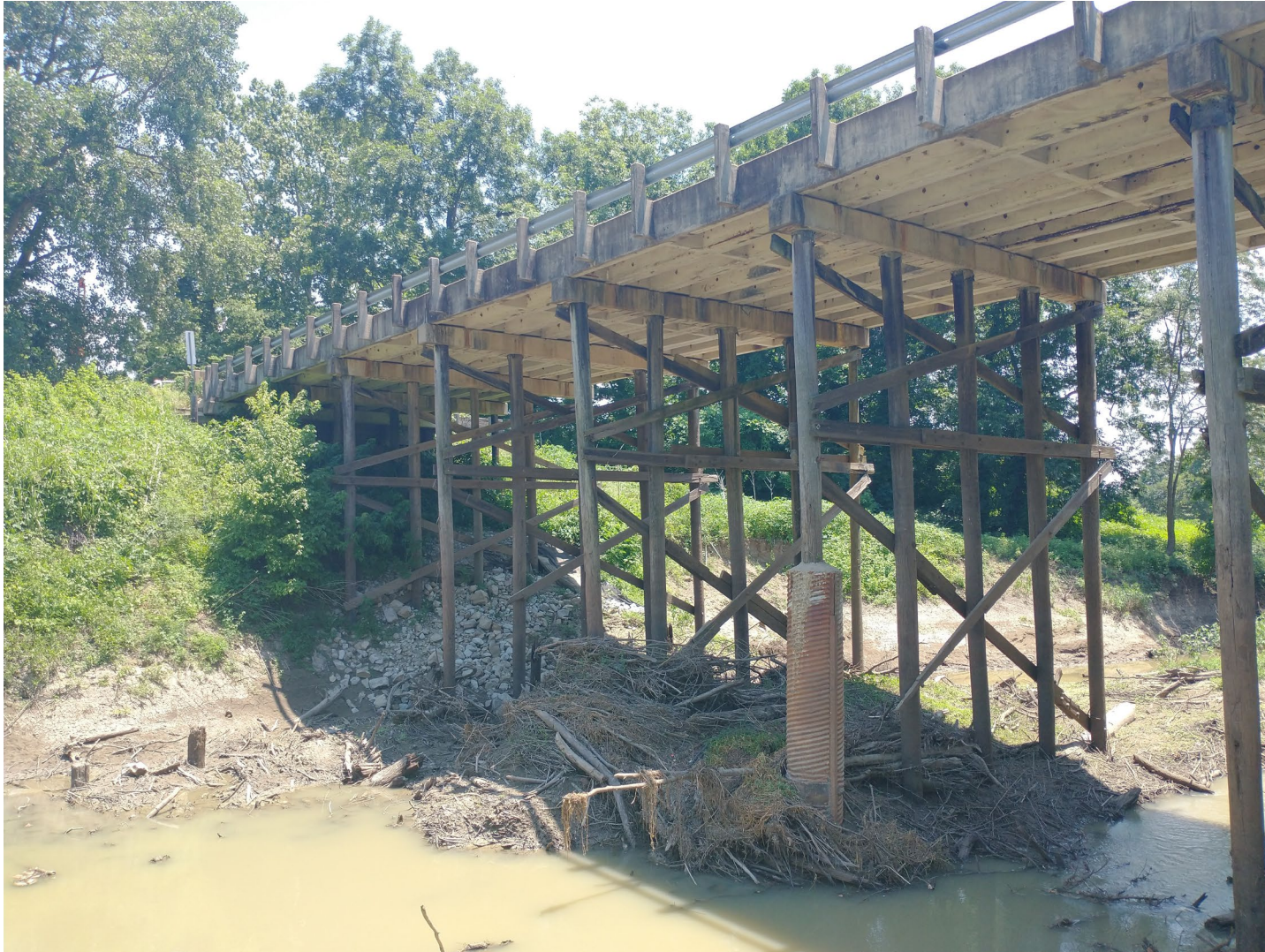
Site 2, Blackfish Bayou (March 2022) Piled up debris on upstream (north side) of the bridge
