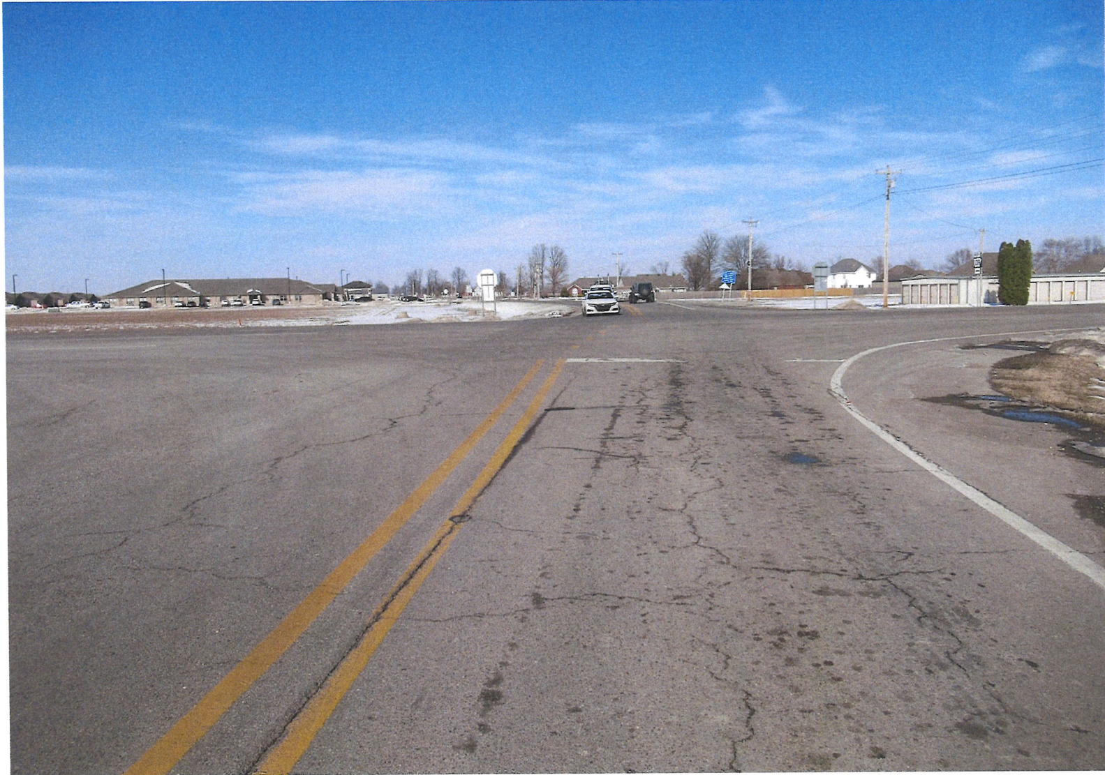
Highway 139 pavement condition, northbound lane.
