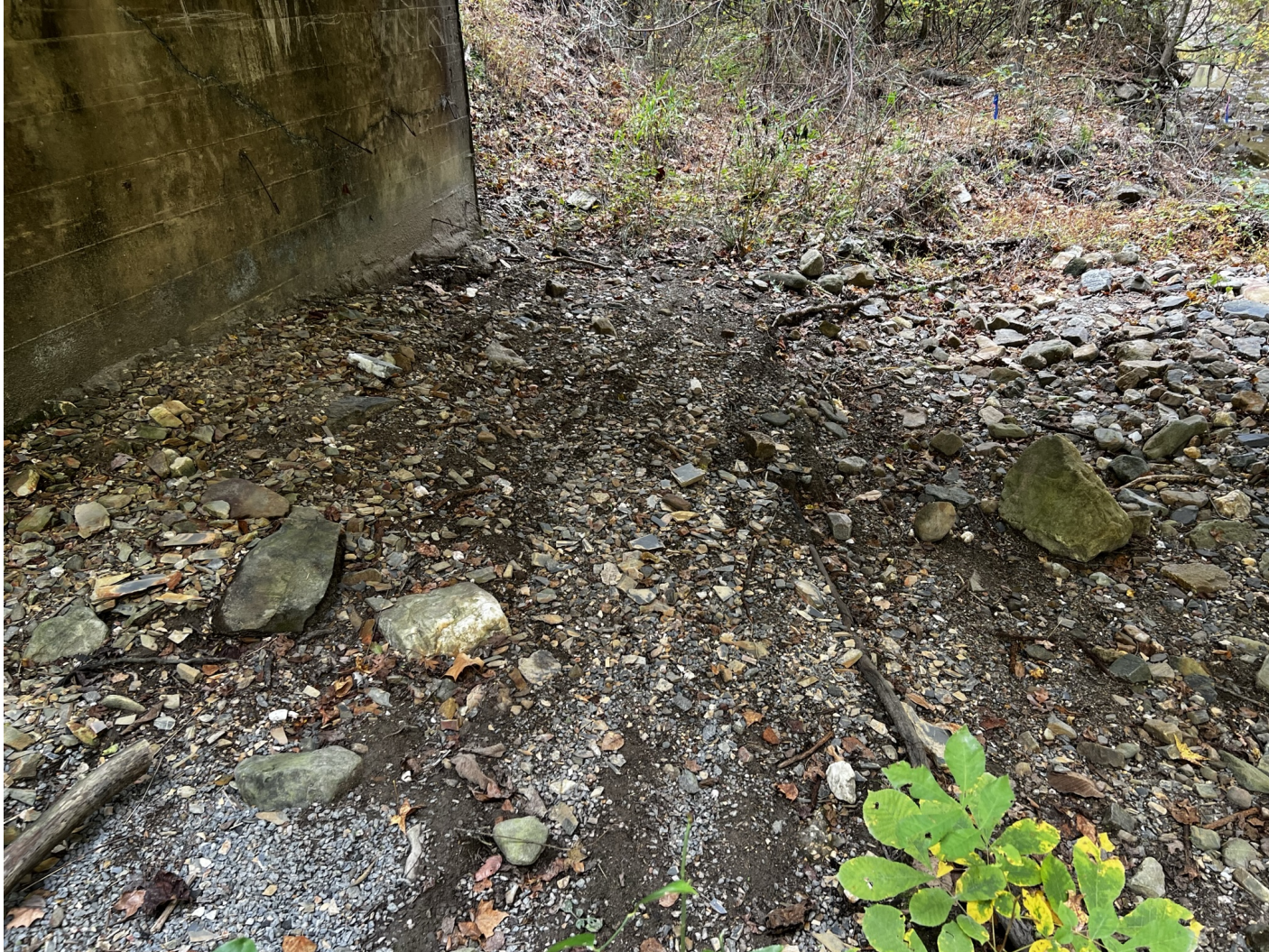
Sediment under south span (October 2022)
