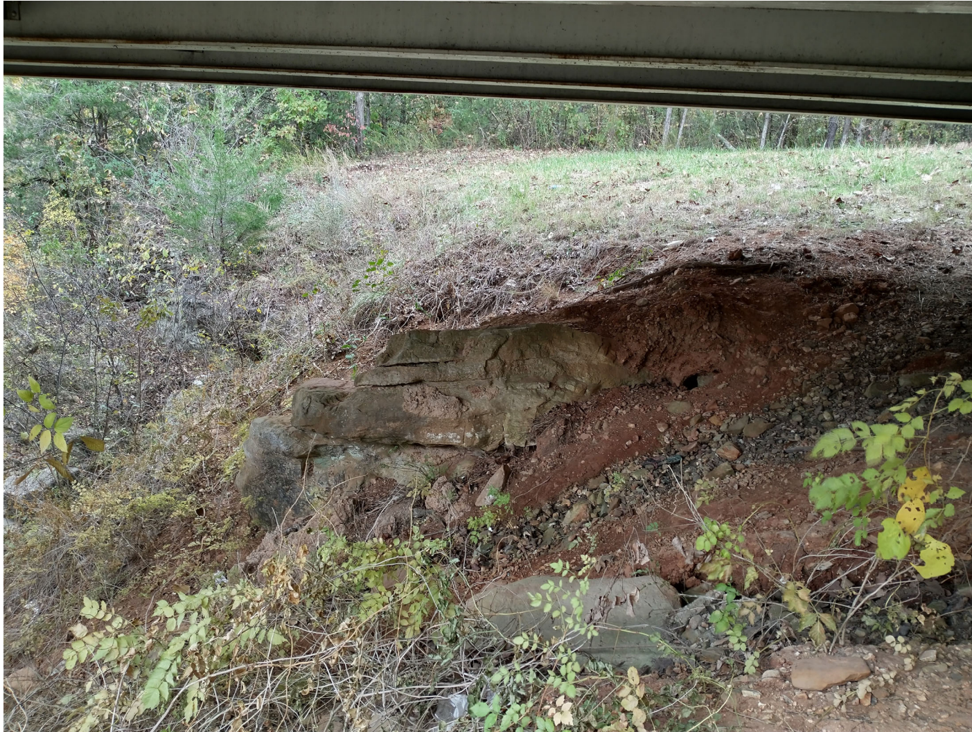
Rock Exposed under West End of Existing Bridge (March 2022)
