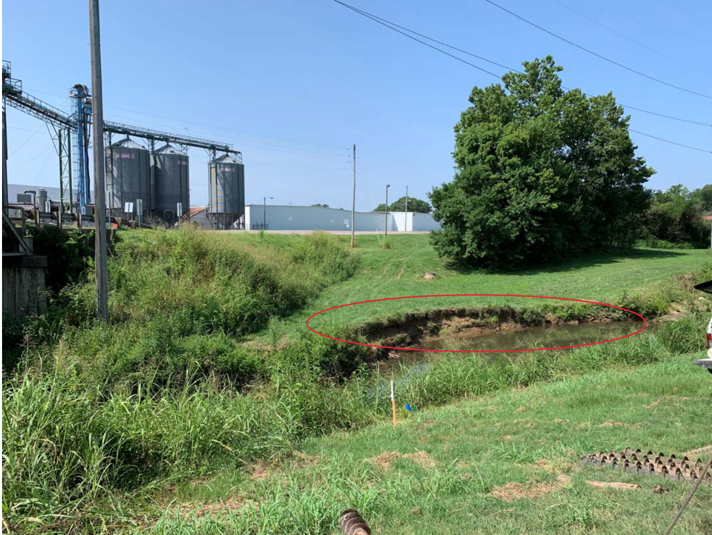
Scour in the Creek Bank - Looking South from North (July 28, 2021)
