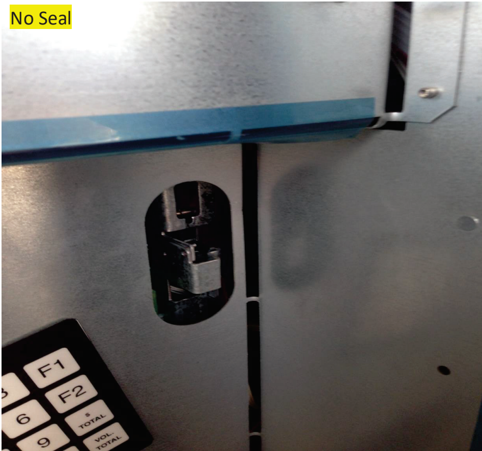
Lead Seal – Must be removed and replaced with state approved seal
