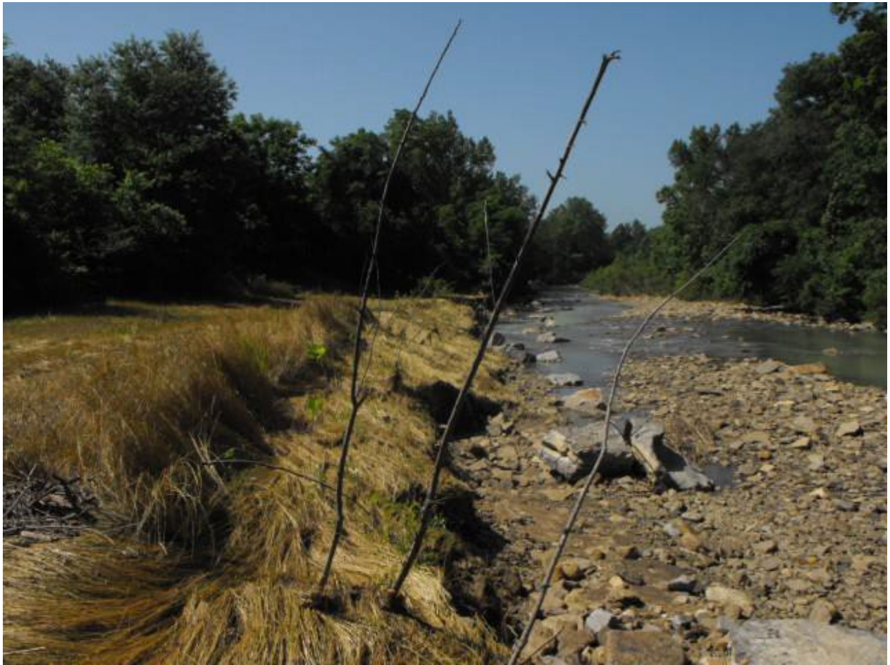
Downstream section post flood.
